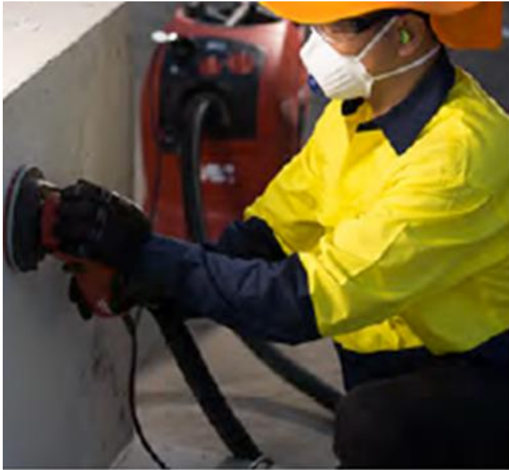
Figure 5: On tool dust extraction (Source: WorkSafe Queensland)
